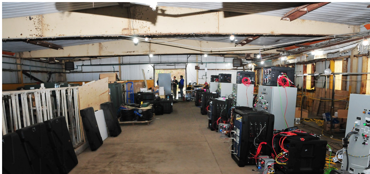
Figure 3.12: PhoenixSEN prototype (black boxes) being evaluated on an electrical grid testbed (gray boxes) in a DARPA RADICS exercise on Plum Island, NY, October 2019. Photo author: DARPA. Photo source: https://www.darpa.mil/news-events/2021-02-23 . Used under the DARPA User Agreement terms.
