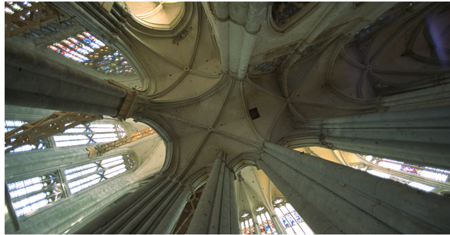
Inside the soaring, 700-year-old cathedral of St. Peter in Beauvais, France, an endangered structure. Maurice S. Luker III / Columbia University
